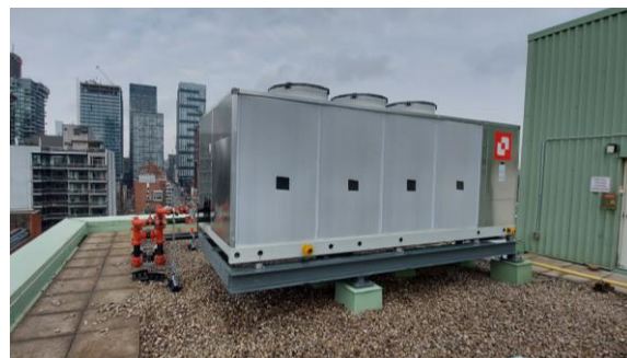
Figure 1. (Top) FQSF consists of two condo buildings sharing a common space heating system. (Bottom) ASHP installed on rooftop.
