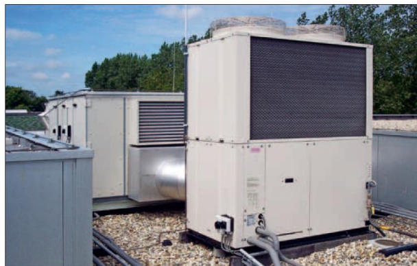
Figure 111: Gas Engine Heat Pump Installed on the Roof
