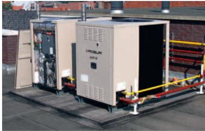
Figure 25: Outdoor Gas Absorption Heat Pump 20
