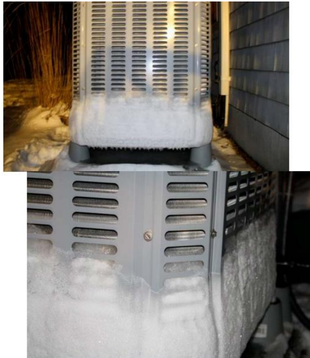
Figure 63: Ice Accumulation on Outdoor Coil (Ice was not removed during Defrost Cycles)
